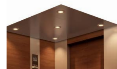
Ceiling: L210S LED downlights (yellow-orange)
